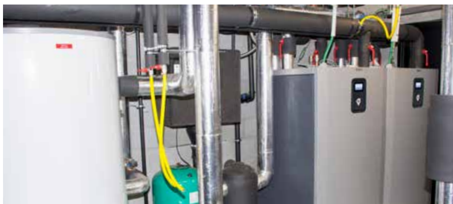
Heating room with two Mega ground-source heat pumps
